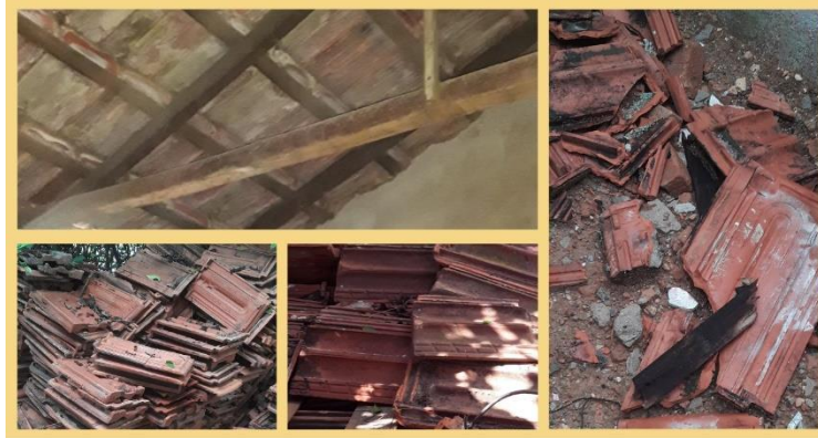
Figure 2. A roof with French tiles (view from below), stock of tiles and on left, some broken tiles.
